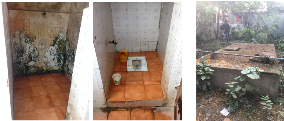
Figure 6: Community toilet in Cuttack- Washing area, toilet seat and septic tank
